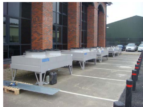
A low energy free-cooling system was specified for the site
