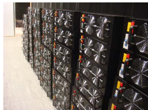
Load bank testing with 4 kW heaters in each rack
