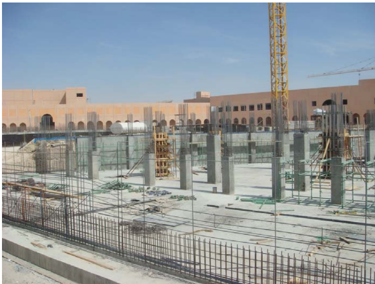
New administration block being built and showing the designated data centre area
