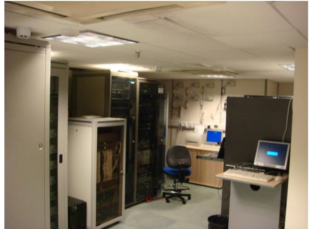
The old 45 m 2 computer room
