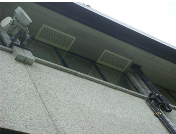
The high level extract and intakes for the air economiser and it's BMS controls being fitted.
